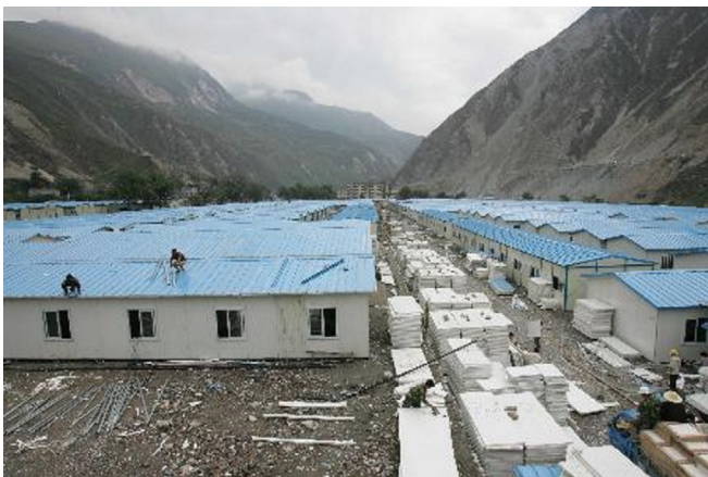
Fig. 1. Prefabricated temporary houses extensively used in disaster relief after the 2008 Wenchuan Earthquake in China.
